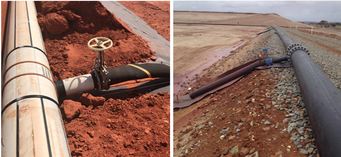
Figure 13: Example of spigot deposition. Spigot at a pre-constructed embankment crest (left) and spigot pipes laid along the main wall (right) (Goldfields, 2023)
