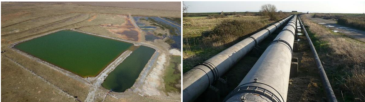
Figure 5: View of a return water dam (left) and residue deposition pipelines (right)
