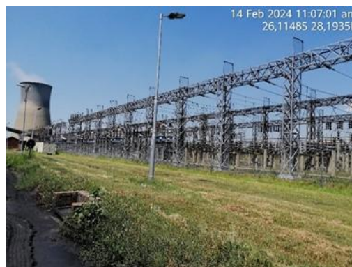
Figure 14: View of the Sebenza switch yard.
