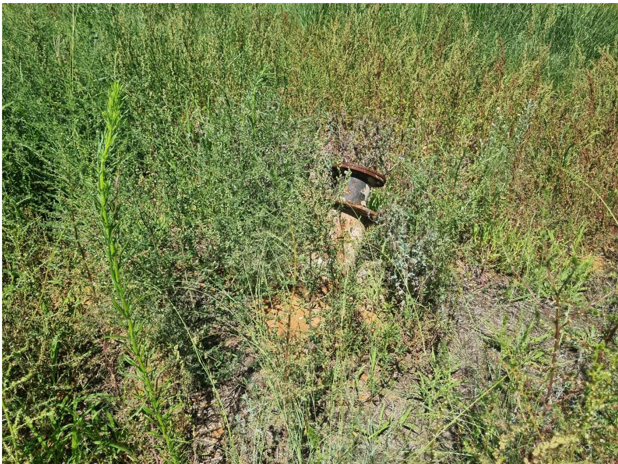
Figure 8: Example of a wellhead in the process of decommissioning, prior to being cut.
