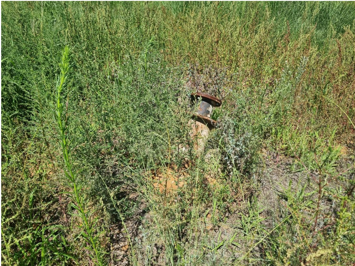
Figure 2: Example of a wellhead in the process of decommissioning, prior to being cut.
