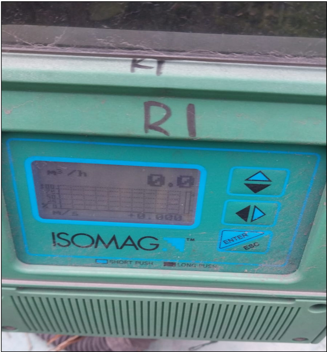
Site Photo 7: Metering Devices across the facility.
