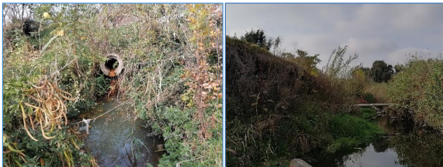
Plate B: Culvert draining unknown effluent into Modderfonteinspruit at site K2 (left) as photographed in May 2024. Sheer banks and bank erosion at site K2 (middle) as recorded in May 2024.
