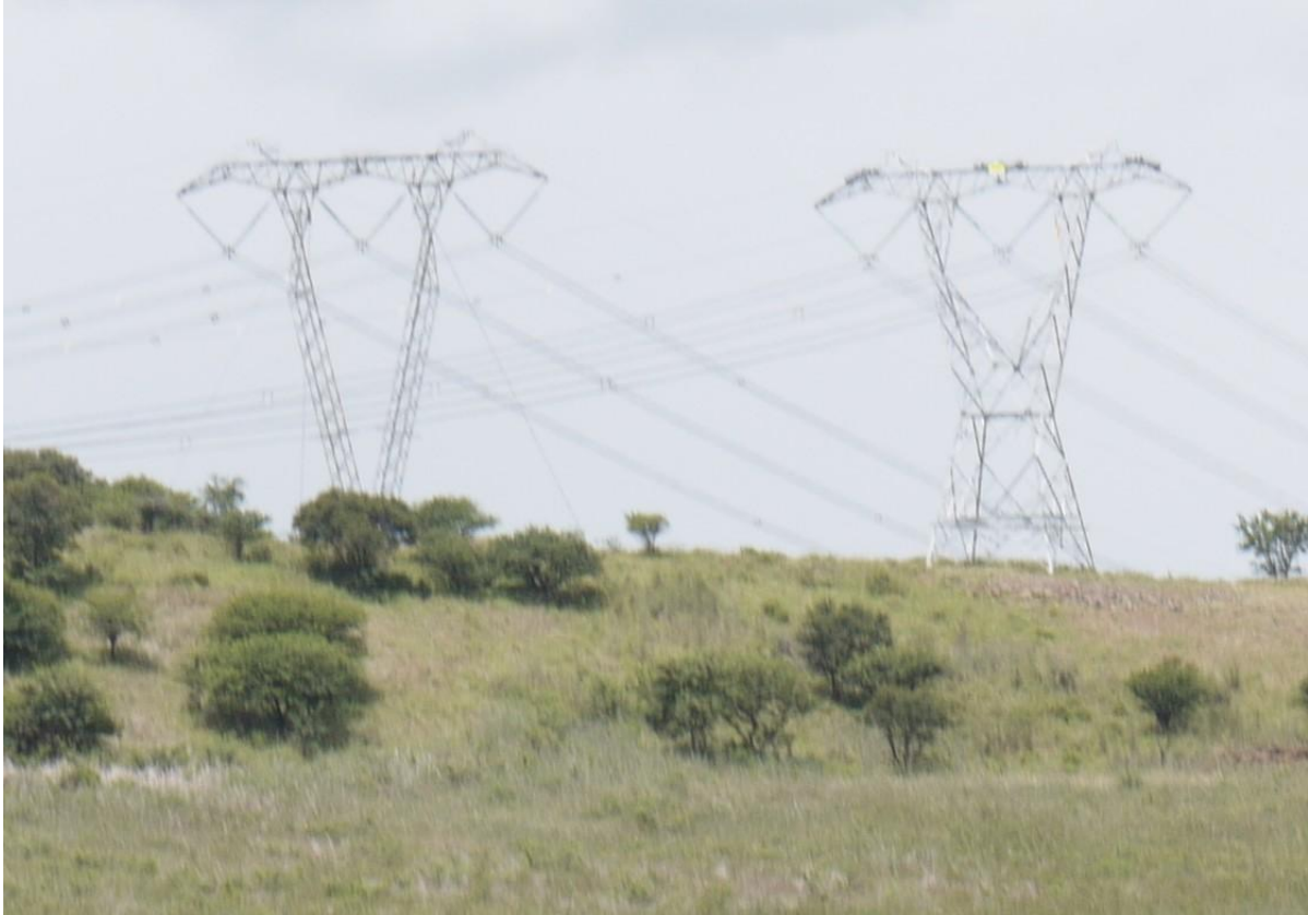
Figure 3: A photograph of the two tower types. Guyed V tower to the left, and cross-roped self-supporting suspension tower to the right.
