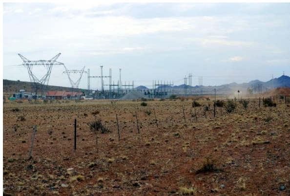
Industrial Landscape Character Area – Paulputs Substation
