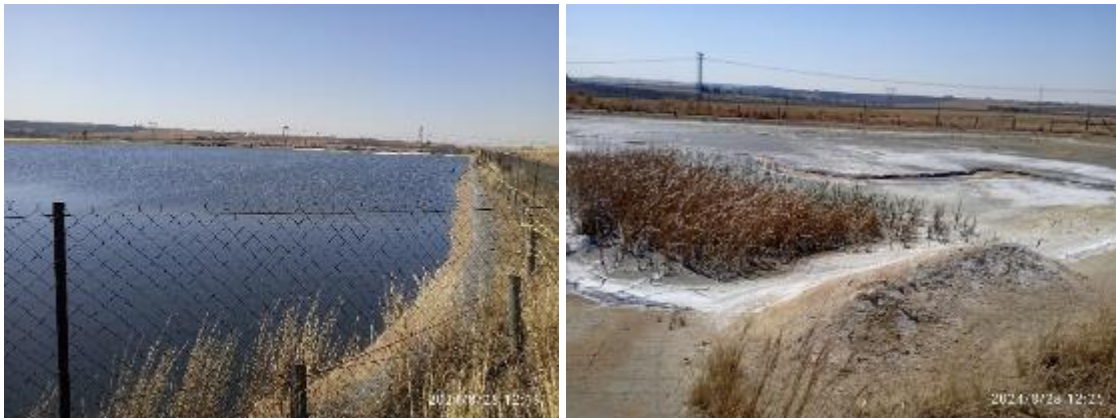
Figure 20: Lined Return Water Dam (34) and poorly maintained silt trap (35) on the northwestern side of Co-disposal facility.
