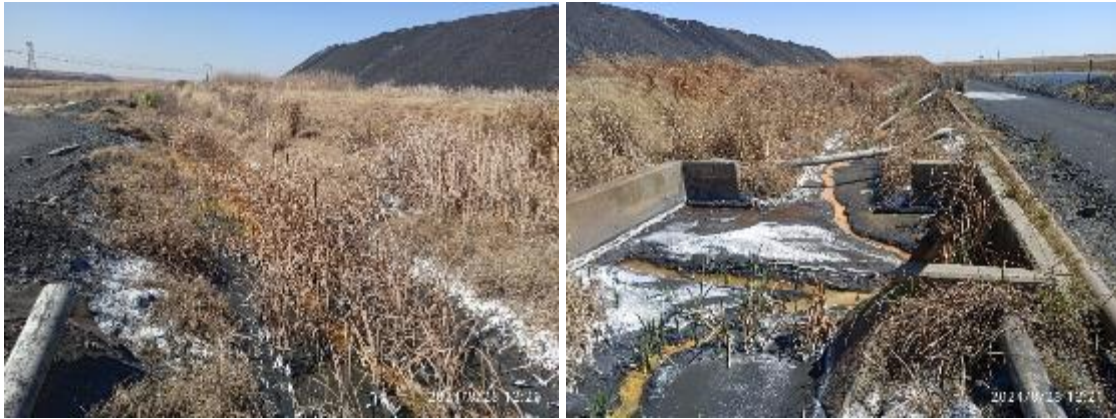
Figure 21: Inadequately maintained north-western drainage system for the co-disposal facility.
