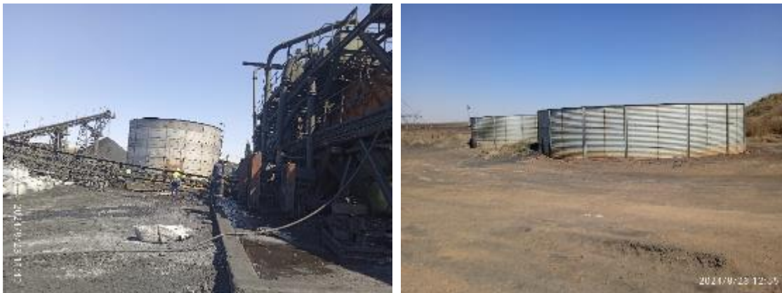
Figure 11: View of Erickson dams at the wash plant (left picture) and decommissioned ones adjacent dam 1 (right picture refer to Figure 2 - 36).
