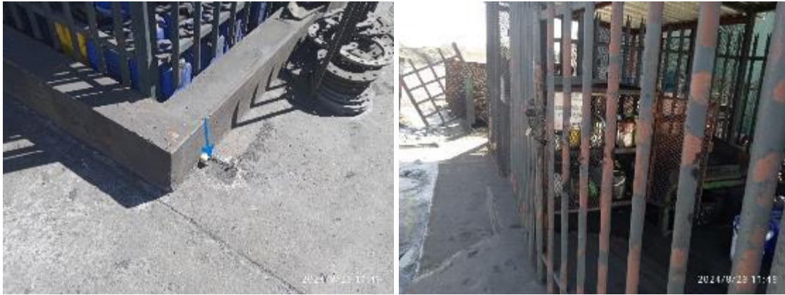
Figure 7: The hazardous storage cage bunded area required a plug on the draining pipe that is open to reduce risk of possible spills to the environment (left picture) and lacks relevant signs (right picture).
